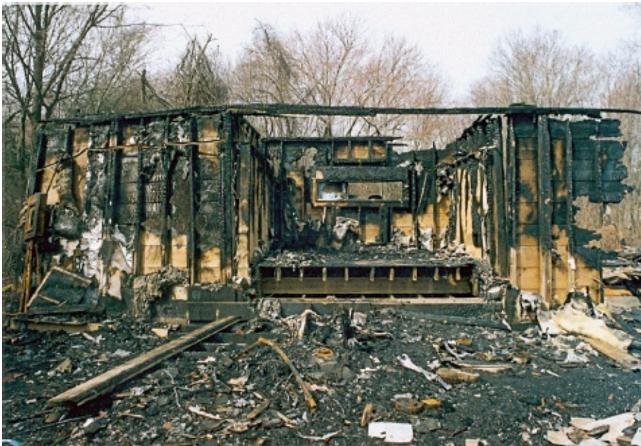
West end of club, post-fire. Remains of stage and drummer's alcove in center
