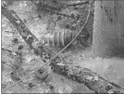
FIGURE 2-3: Little Rock, AR, December 29, 2000. Downed power cables are among the damage after a recent ice storm. (Photo by John Shea/FEMA News Photo.)
